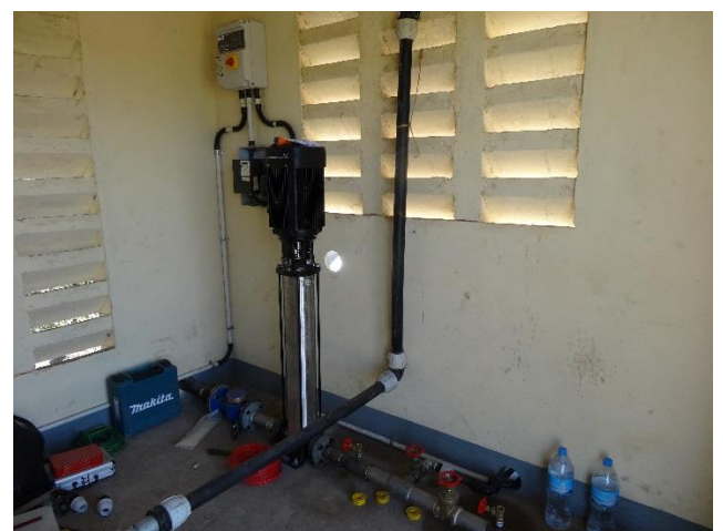
Phase 2 Booster Pump supplied and installed.
